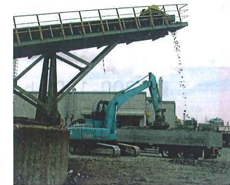
A conveyor drops clean shredded ferrous onto the ground from where it is lifted and loaded by magnet into trucks.
